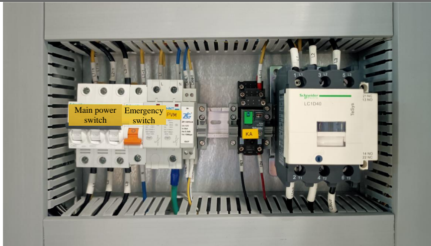
Figure 2.5 Main power switch
